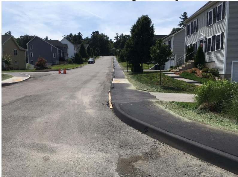
Wachusett Woods sidewalk, curbing, and curb cut ramps project. The Highway Division also installed the final layer of pavement.
