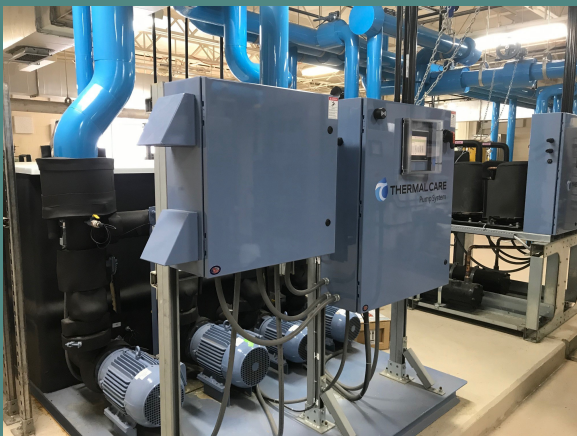
The plant's new controlled system pumps.
